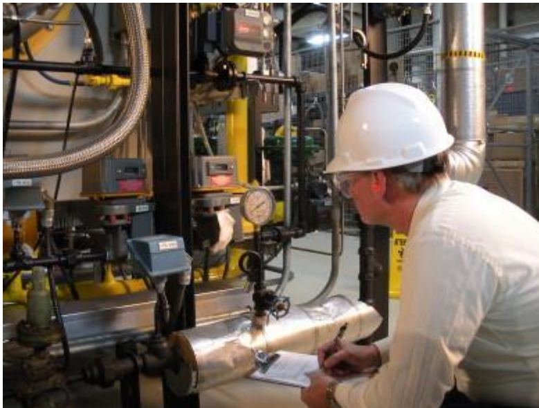
Figure 33: Energy auditor at work
